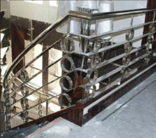
SS Design Handrail at JBR Hilton, Dubai
