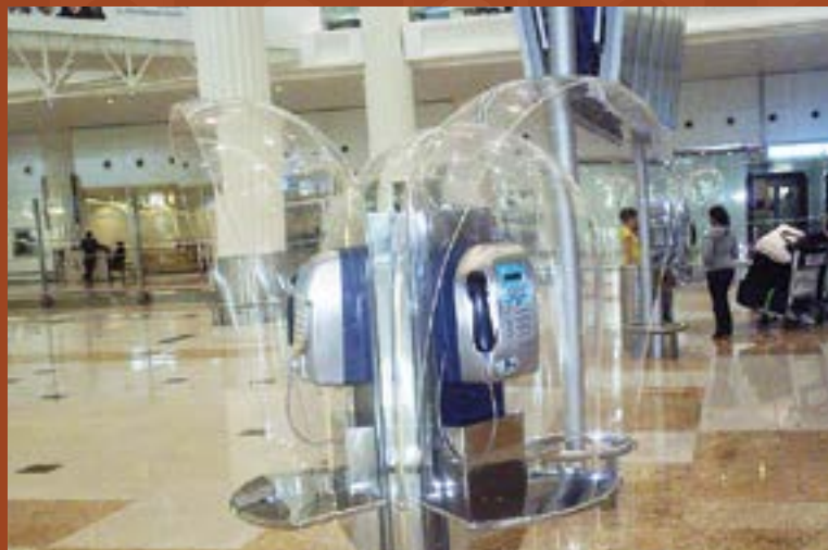
Telephon Booth at International Airport Terminal-3
